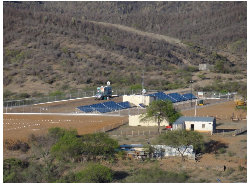
Hybrid PV Systems and Mini-Grids Fraunhofer ISE
